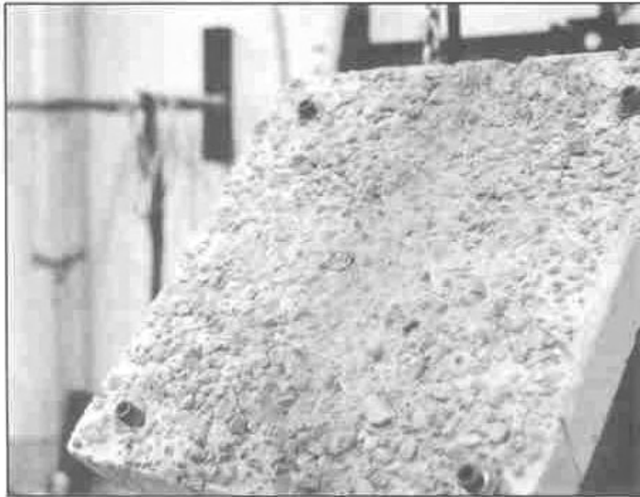
Figure 2: Rough concrete slab with small pebbles embedded into the surface (see penny for size comparison to pebbles).
